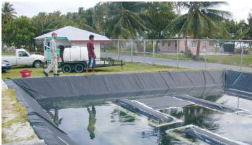
A water treatment plant, part of an ADB project to improve water and sanitation facilities.
